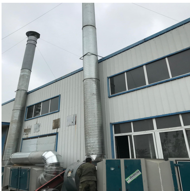
2套“过滤棉+活性炭”装置+2个15m高排气筒
